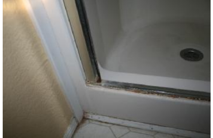
2. Metal corrosion and water leakage around the metal frame of the shower door. The door and
