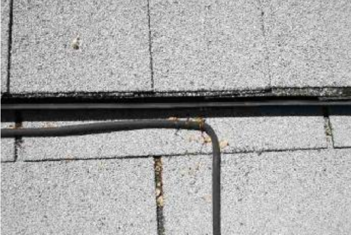
1. Staples were used to secure the TV cable near the ridge. Potential leak area.
