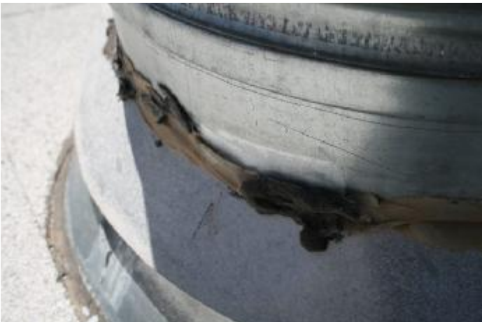
5. Silicone and tar sealant should be removed and replaced with an appropriate sealant. All
