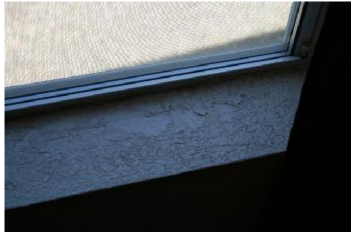
4. The North Family room window has evidence or rain/water damage. This should be
