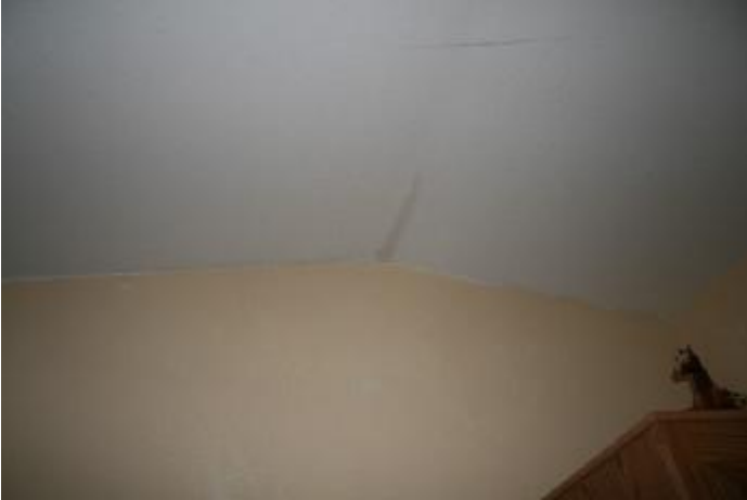
1. Dry wall settling cracks. Master bed room.
