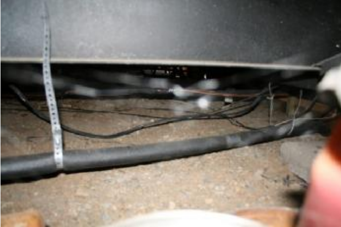
1. The crawl space was inspected at the access door only, due to it's limited access. Supply
