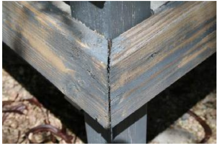
4. Wood at the front and back entry roof shows evidence of cracking, delamination and dry rot.
