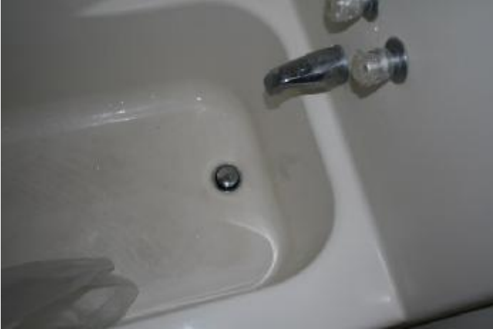
1. The guest bathroom tub drains slowly. The requires further investigation to determine if it
