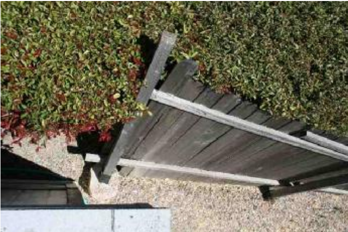
5. The front fence is in need of repair.
