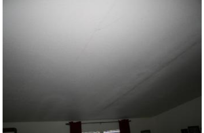
2. Several drywall cracks in the front room were noted. This could be normal settling but needs
