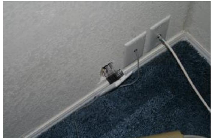
6. The wall plugs for the internet connection are loose and falling out. They should be properly
