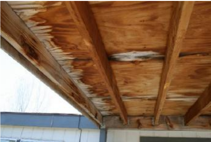
3. Underside of the front entry covering showing evidence of past water damage.
