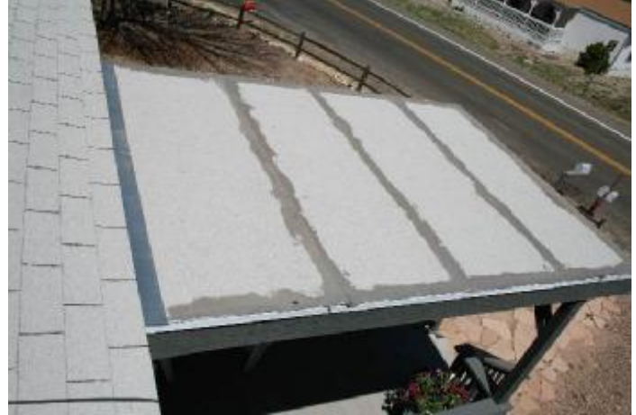
2. Attached covered entry leaks at the house and the entire length of the covering. This
