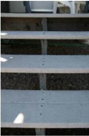
3. Screw heads should be level with the step plank surface, a potential tripping hazard. Cracks
