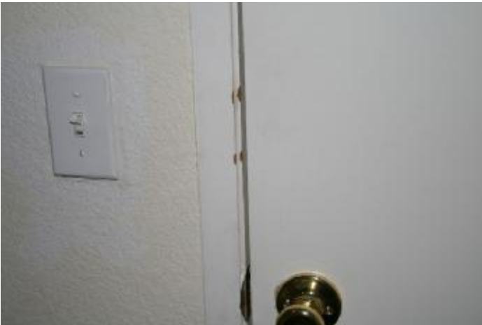
3. Several of the doors close but do not latch. The strike plate needs to be adjusted to ensure
