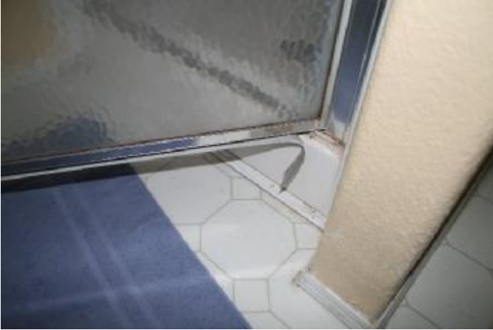
3. Water seal separating from the shower door.
