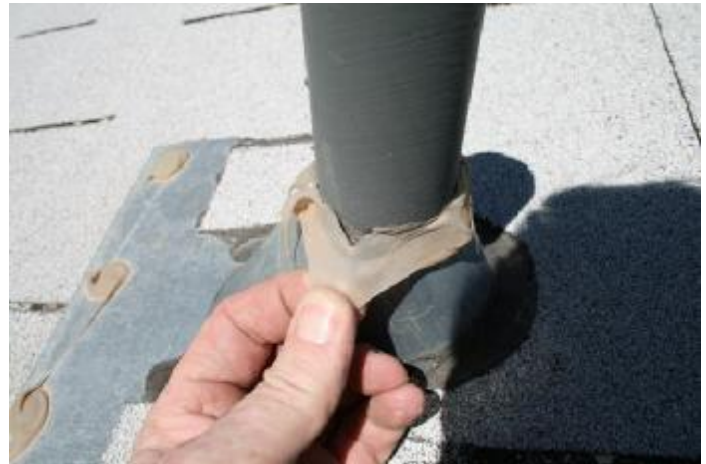
4. Loose silicone no longer forming a seal around the vent pipe. Roof flashing should be
