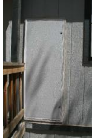
2. Access to the water heater was denied at the time of inspection due to the locked door. It is
